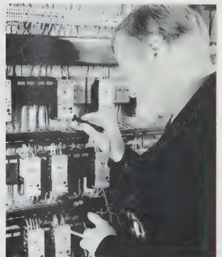
A technician checking control panel operation as part of preventative maintenance procedure.
