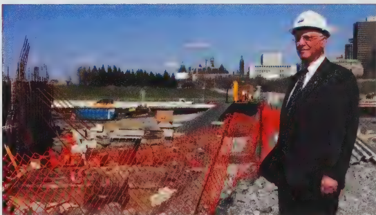
It's full speed ahead as Paul Manson, Sc'57, chair of the $15-million fundraising campaign for the new Canadian War Museum, surveys the Ottawa job site.
