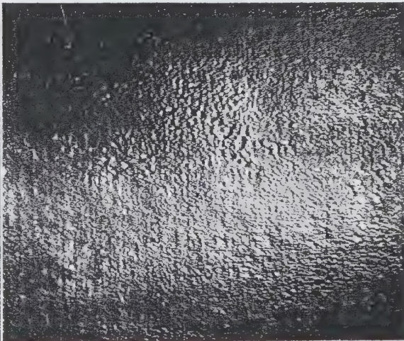
Figure 5. Detail of pitted paint surface.
