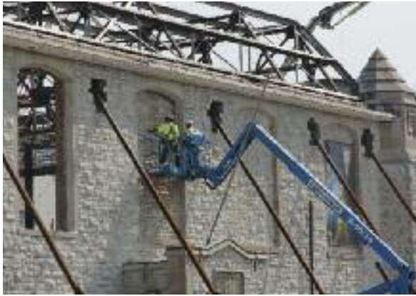
Workers are tearing out stone that has filled these window frames since 1970. New heritage-style glass windows will be installed by December.
