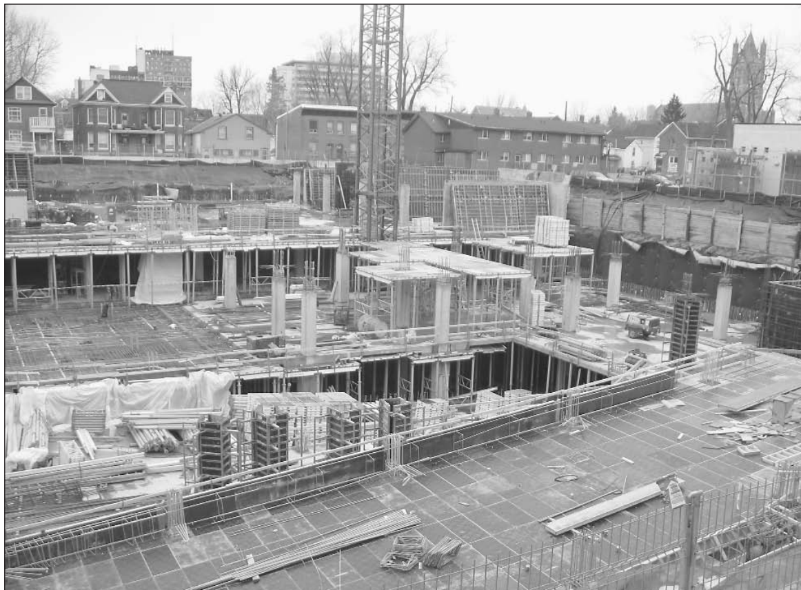
A view of the Queen's Centre construction looking north-east toward Earl and Division streets.
