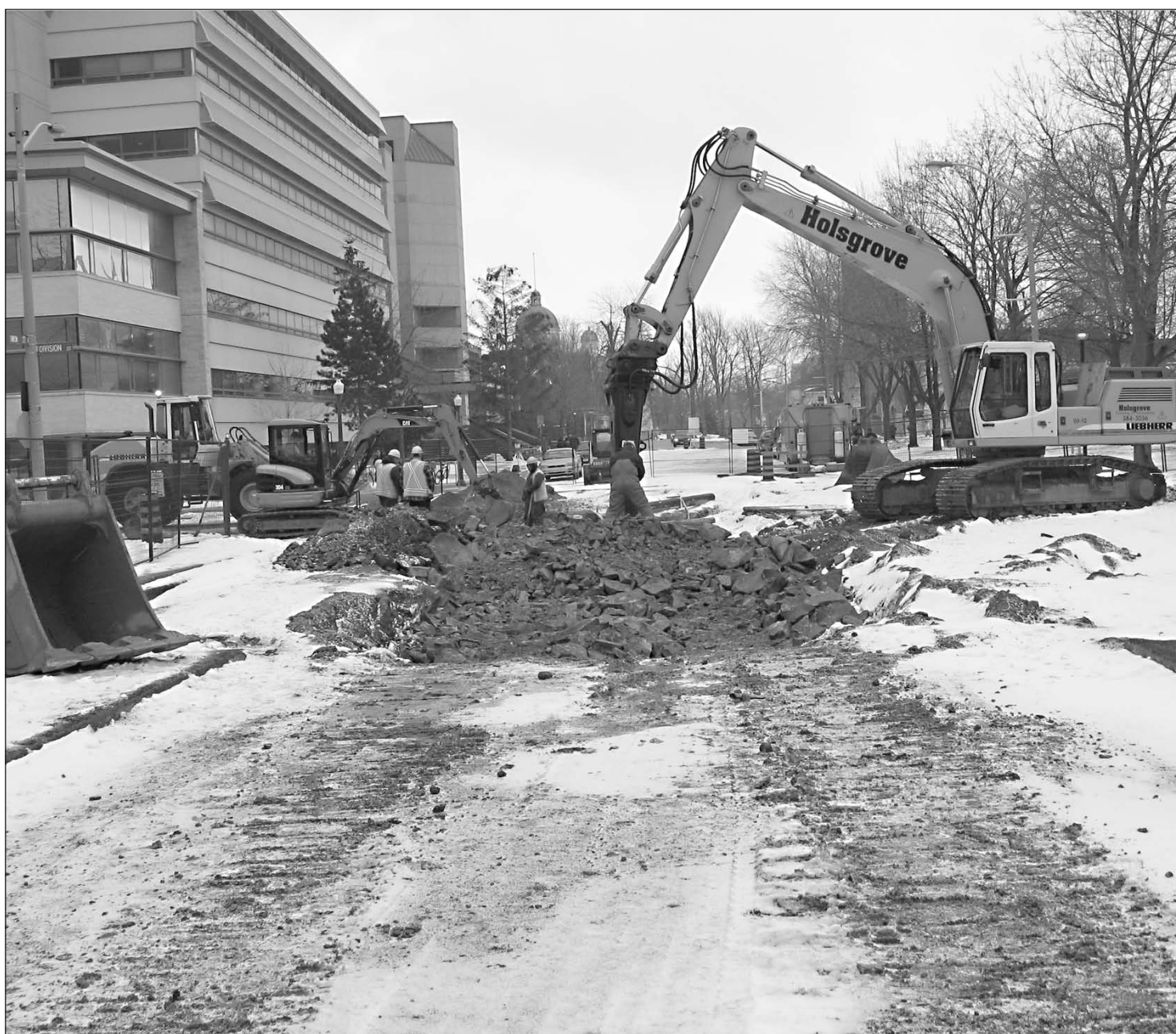
Workers begin excavating Union Street at Division Street to allow for the rerouting of site services, water sewer and electrical, for the Queen's Centre project. CELIA RUSSELL
