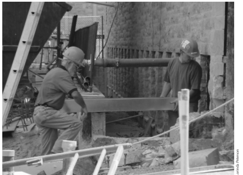
Workers carry building material at the site of the new entrance to Macdonald Hall. Renovations, which are to be completed this fall, include a new elevator and other accessibility improvements and improved building presence.
