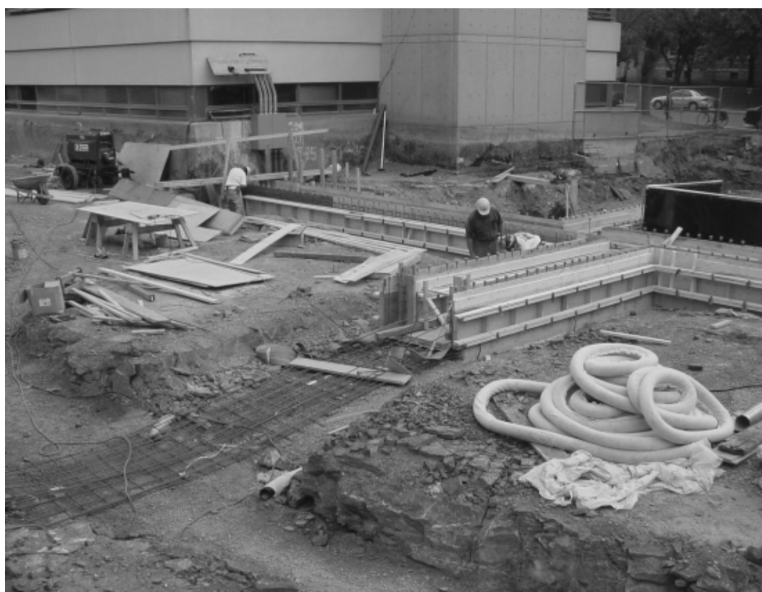
Laying the foundation for learning. Construction workers work on the foundation of the Integrated Learning Centre at the corner of Division and Union streets between Goodwin (shown at rear) and Dupuis halls. The building is scheduled to open in January, 2004.
