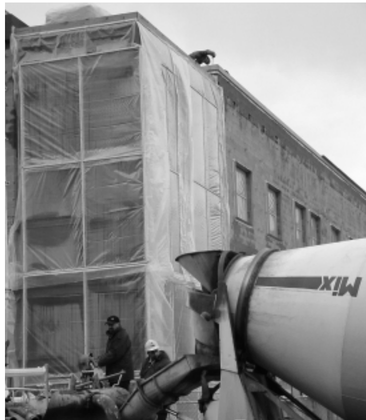
Pour it on: Workers pipe cement into an upper floor of the new School of Business building on Alfred at Union streets last Thursday. Goodes Hall is scheduled to open officially this September.
