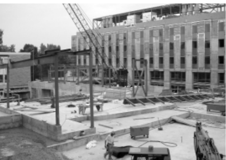
Work continues on Chernoff Hall, home of the new chemistry building, on Queen's Crescent. The facility is slated for completion in Spring 2002.
