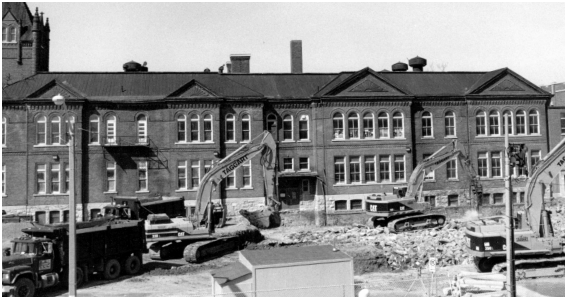
Heavy equipment begins drilling and digging for the addition to the former Victoria School, soon to become Goodes Hall, new home of Queen's School of Business. The renovated and expanded facility is slated for completion in May, 2002.
