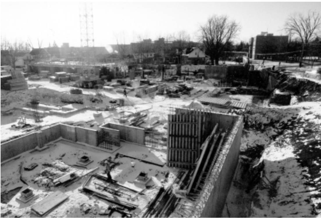
Firm footing: Work on the foundation of the new Chemistry building, Chernoff Hall, on Queen's Crescent continues in the snow. The building is slated to open in spring, 2002.
