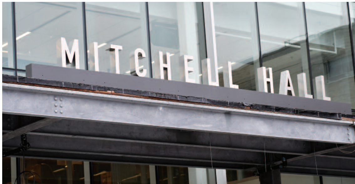
As construction continues at Mitchell Hall, the eastern entrance now bears the name of the building's lead donor.
