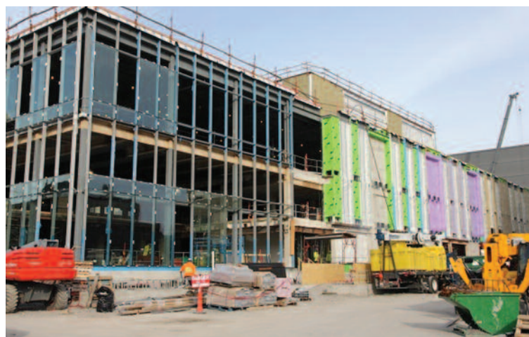
Heavy pre-cast concrete panels are lifted into place on the north side of the Innovation and Wellness Centre. The panels are being trucked in from Ottawa.
