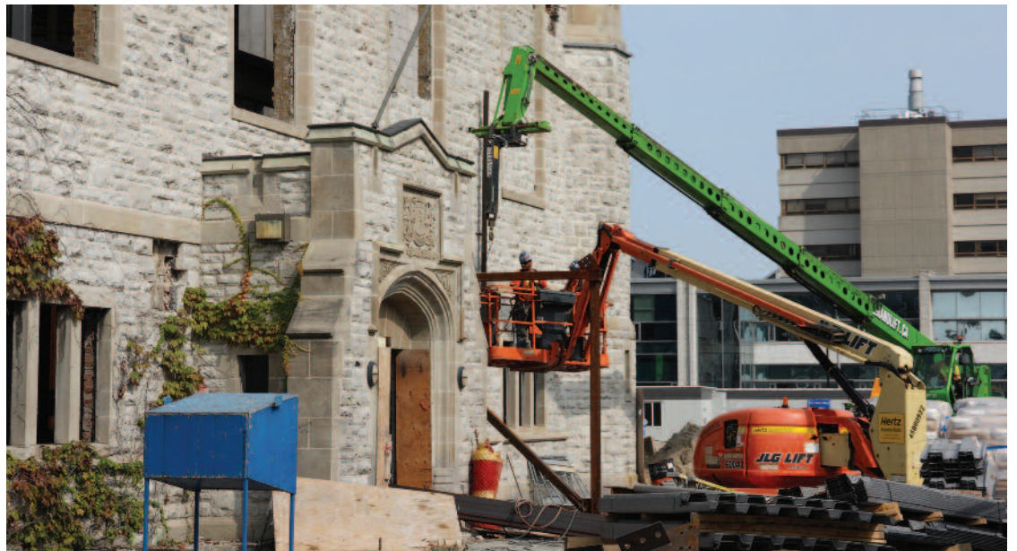
Workers remove the final piece of shoring from the front facade of the Innovation and Wellness Centre as construction of the facility continues. The construction site is scheduled to be enclosed by the end of 2017.
