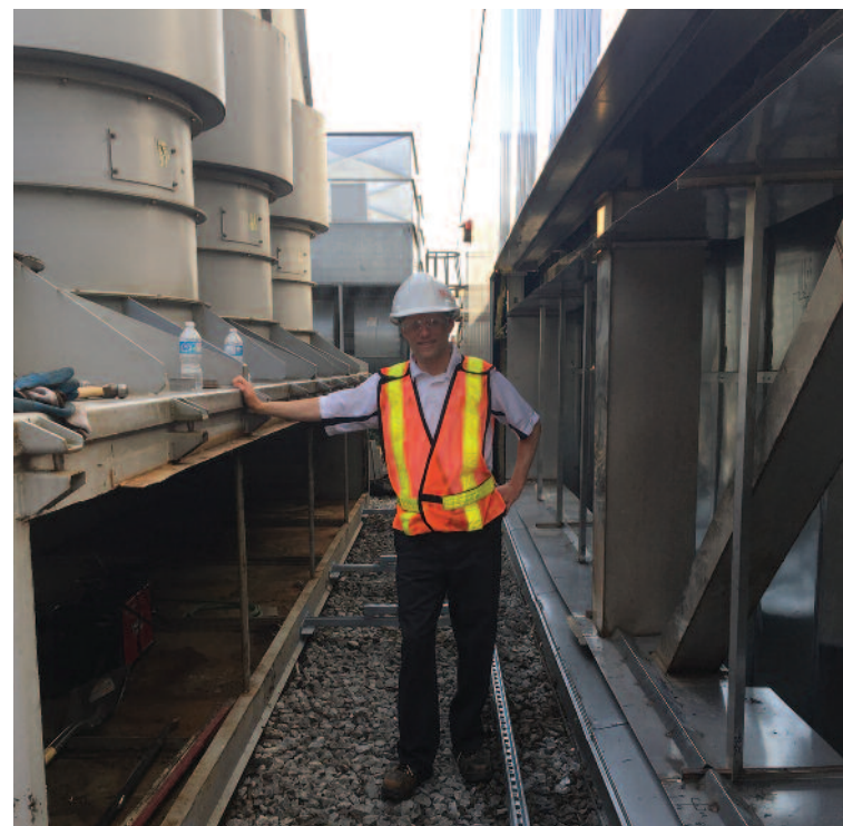
Nathan Splinter, Energy Manager for Physical Plant Services, stands beside the new heat recovery glycol coils that have been installed atop Chernoff Hall.
