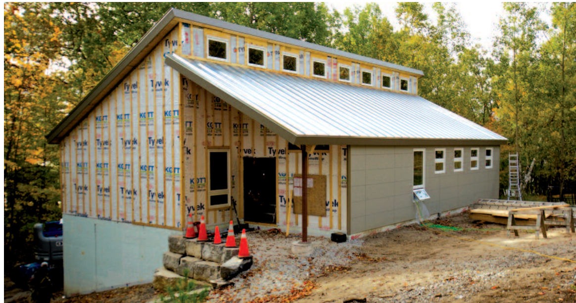
A $1 million gift from Jessie Deslauriers', Artsci'87, Artsci'91, is resulting in the construction of a new research and teaching facility at Queen's University Biology Station (QUBS).
